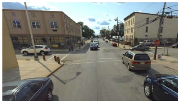
Faded crosswalks and center lines on High Street (top) and Fayette Street (bottom)
